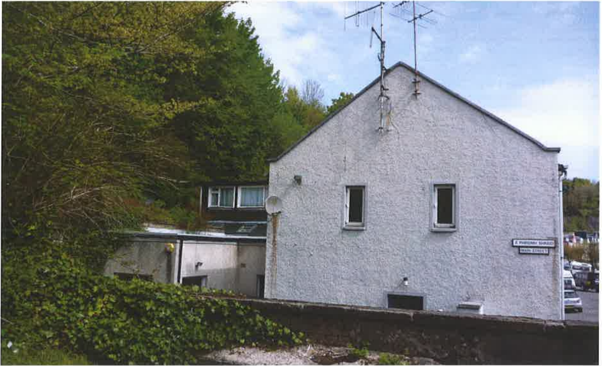
Figure 5 : Timber Clad, Profiled metal roofed extension to rear of building on Main Street, visible from main road
