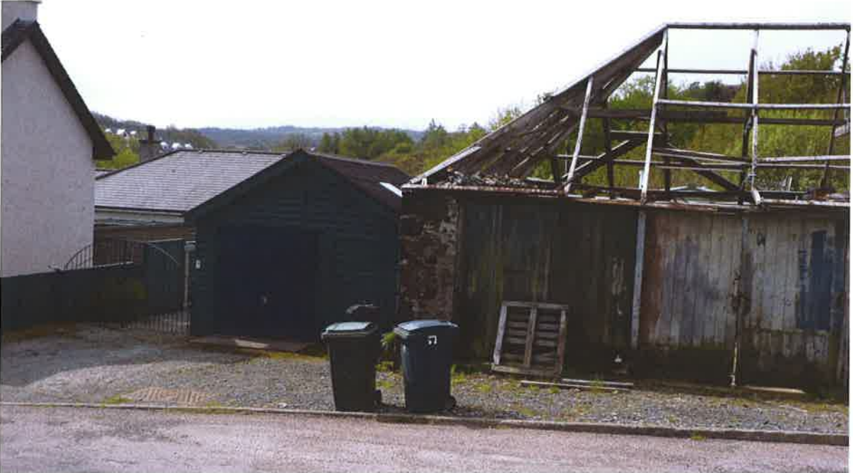
Figure 19 : Timber Garage with corrugated roof (beside, until recently, metal roofed building) on main street scene
