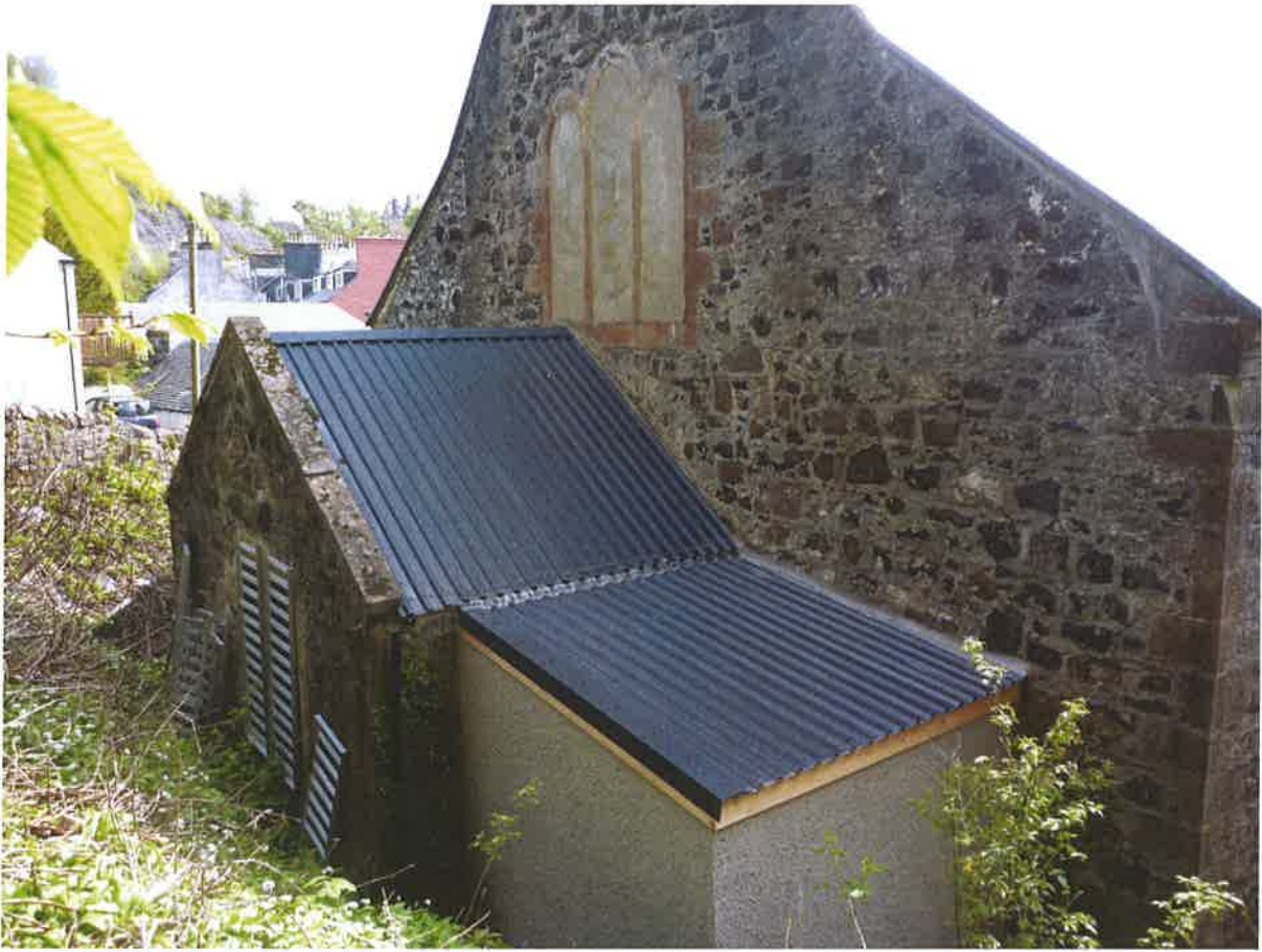
Figure 4 : Profilled Metal sheet roof on Listed Building (the Gallery) on Main Street
